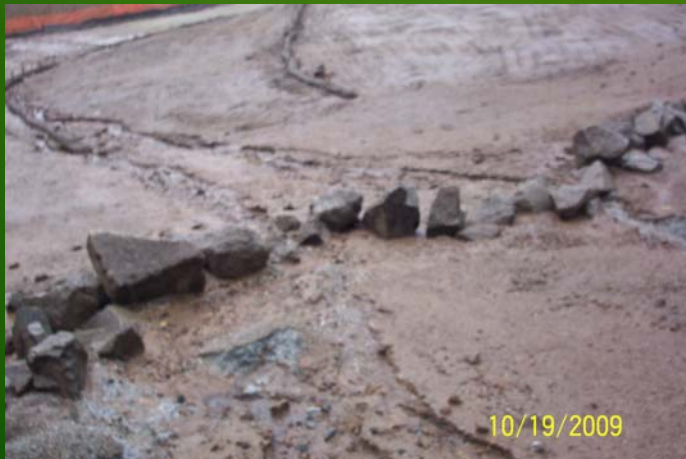
Infiltration ditch overwhelmed
