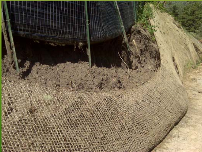
Hillside blowout on horse trail
