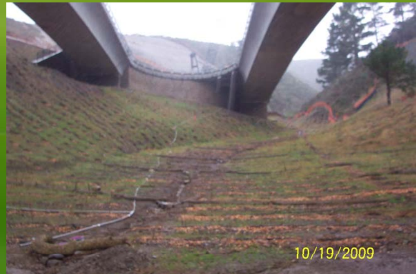
Rilling at swale
